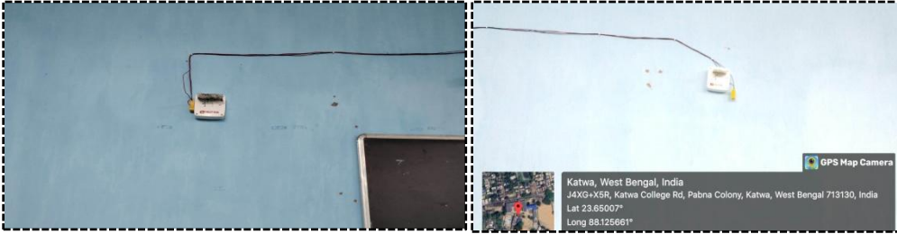
Sensors mounted on the wall of class rooms
