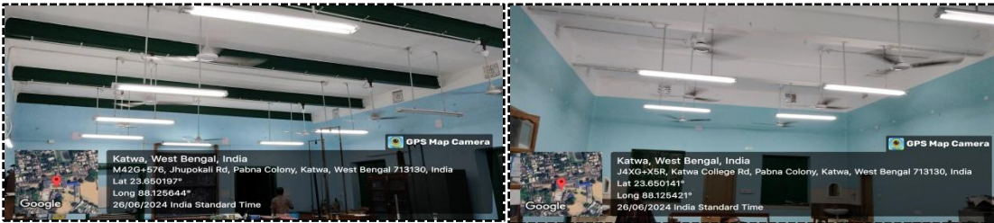
LED facility in the class room
